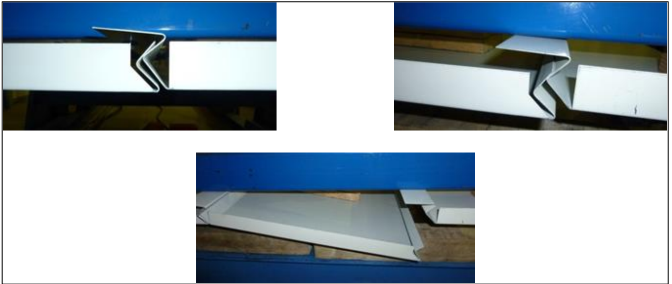
Figure 1.4 Gradual dislocation of the joint during suction loads tests
